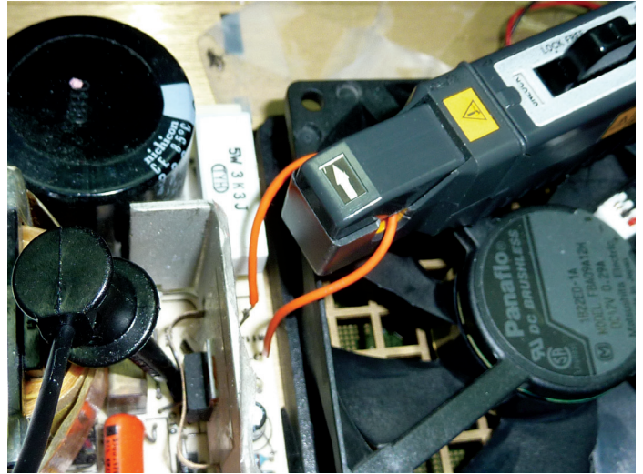
Figure 4. Creating a special current loop in your power supply to measure current.
